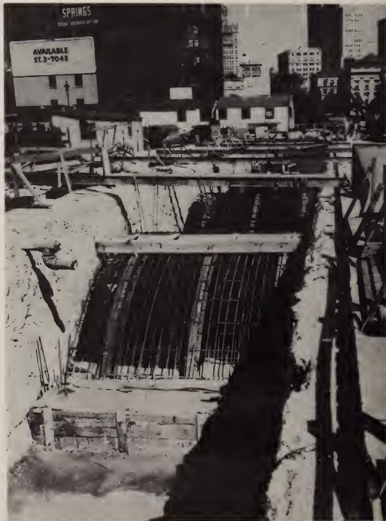
Reinforced steel is ready for the new arches over the north subway cut.
